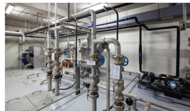
Greywater/stormwater system: Collect rainwater and underground water on the building rooftop and on the ground to reuse as raw greywater or landscaping water
